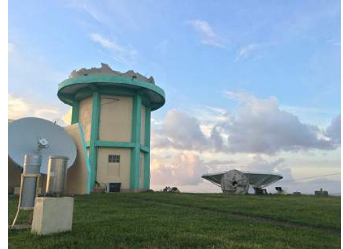
Destroyed PAGASA Radar Dome
